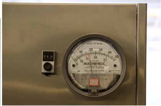
Pressure gauge for airflow
